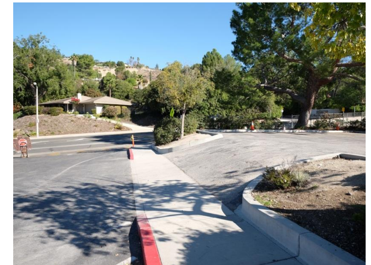
Photo -2 Driveway up to secondary parking needs to be repaved to correct slope to avoid damage to both the cars and the driveway.
