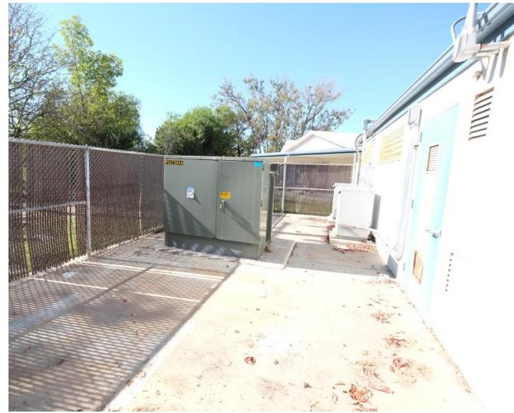
Photo 26 Building Name: N/A Building Number: N/A Utility units behind Building 5.
